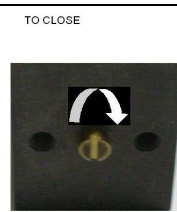
Manual Override "ON " Photo - 6
