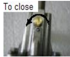
Manual Override "ON" Photo - 3
